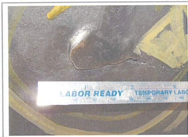
Photo reference of MFG Defect in piping
